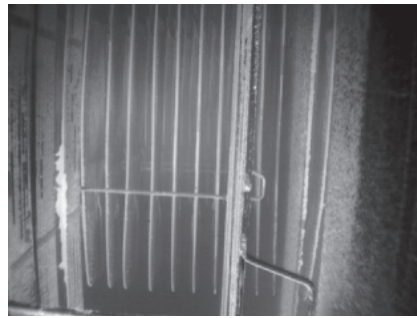
Superheat pendants in 700MW power boiler burning PRB coal
